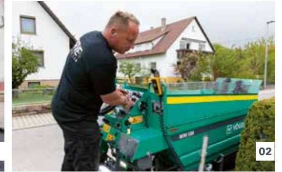
01 MINI pavers are outstandingly suitable for paving asphalt between tracks or in milled tracks. 02 MINI pavers are the first choice wherever space is at a premium.
